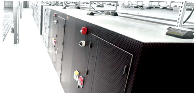
IO's Next-Generation Modular Data Center
